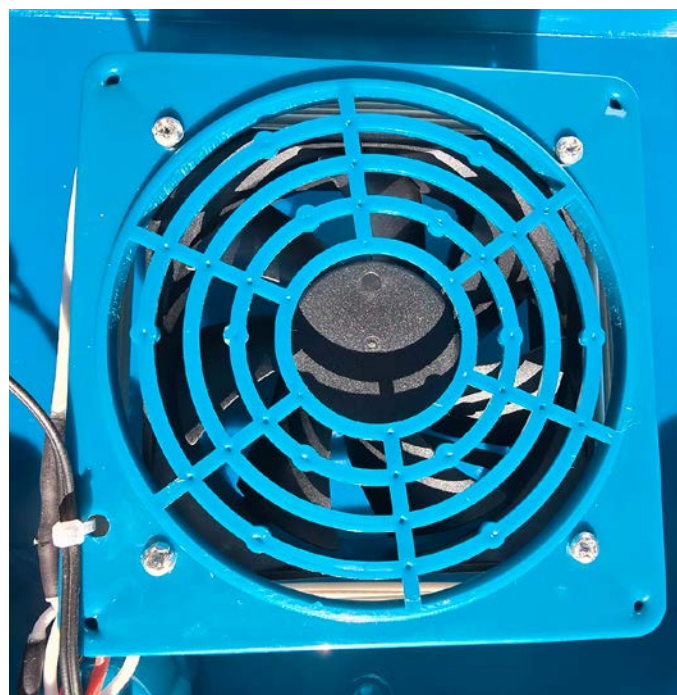
The fan would be impossible to clean as the screwheads had been fouled
